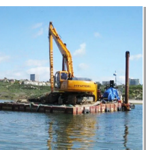
Floating Barge 150 ft x 36 ft x 07 ft
